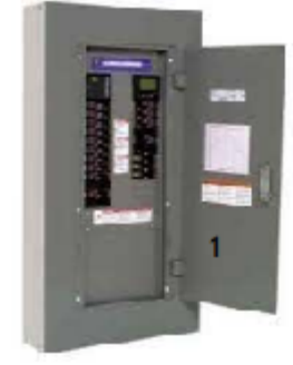
Building Electrical Panel
